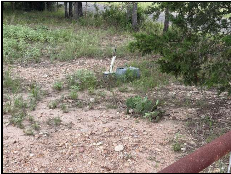
12. Water Meter On CR 216 Which Service Cabins.
